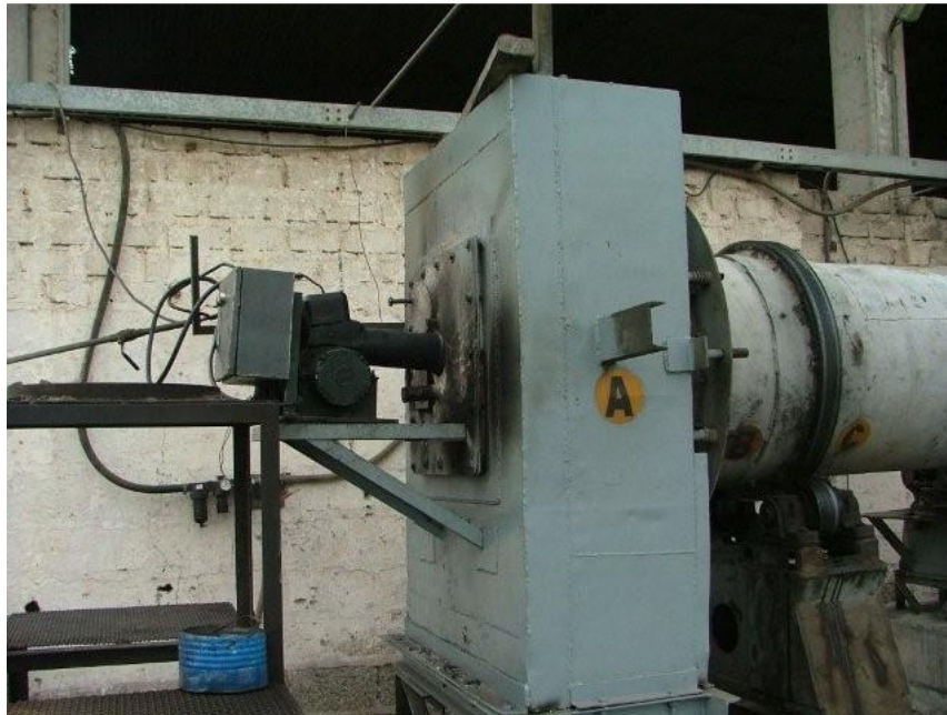
Figure 8 : Gas lance on slag end of kiln
