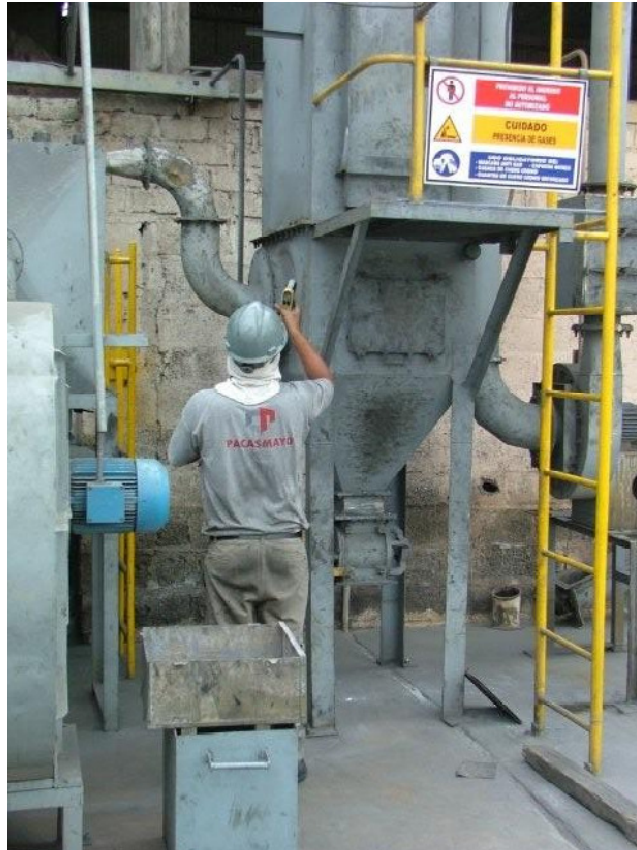
Figure 5 : Monitoring the temperature in the baghouse
