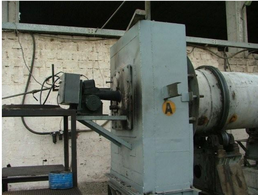
Figure 7 : Gas lance on slag end of kiln
